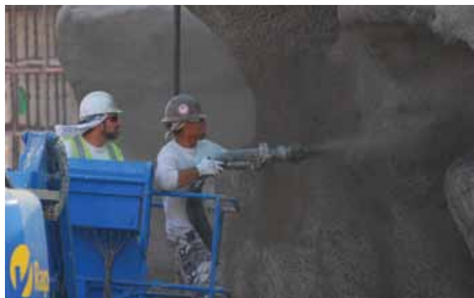
Workers place shotcrete for rock formations; Al Ain Wildlife Park and Resort, Al Ain, UAE
